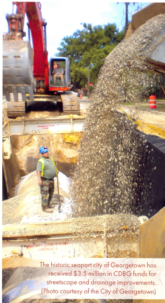
Workers in Wagener repair damages to their aging water/sewer infrastructure, thanks to CDBG funding (Photo courtesy of Mayor Michael Miller)
